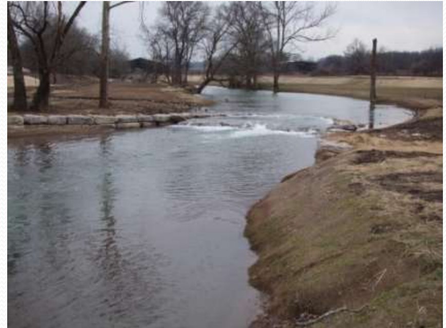
Restoration of Murfrees Fork of the West Harpeth River , Williamson County, TN (during construction)
