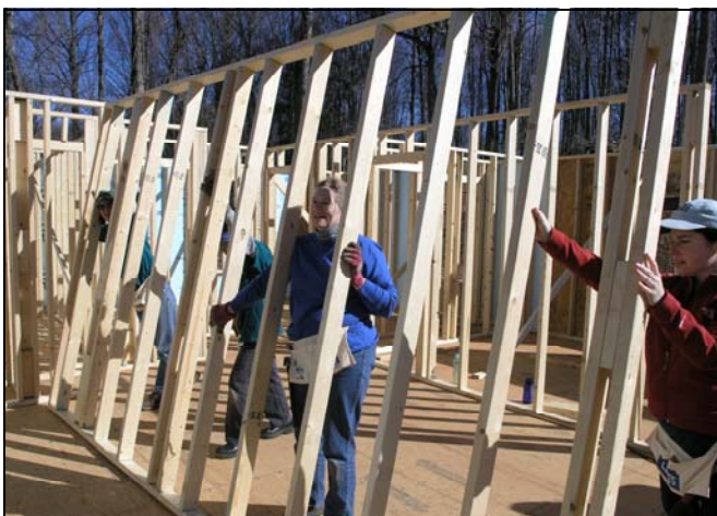
2007 Women Build volunteers raised interior walls about a week into the project.
