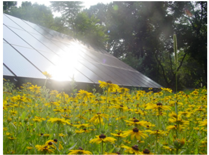
Figure 8. The solar photovoltaic array at The Schuylkill Center provides financial and environmental benefits and is an educational tool as one of the Center's permanent exhibits.
