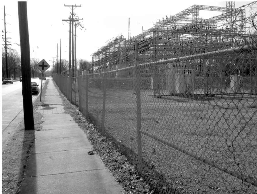
View substation along 14th Avenue South
