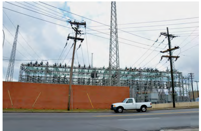
View of substation from school parking lot on Dr. DB Todd Jr. Boulevard
