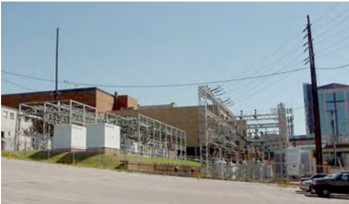
Substation at Broadway and 10 th Avenue, Nashville
