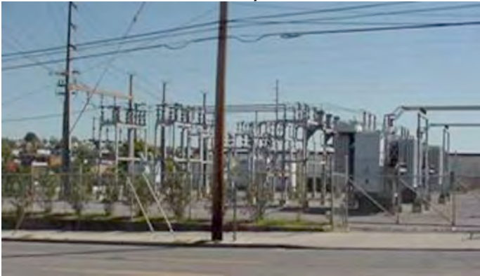
Substation at Demonbreun and 6 th Avenue, Nashville
