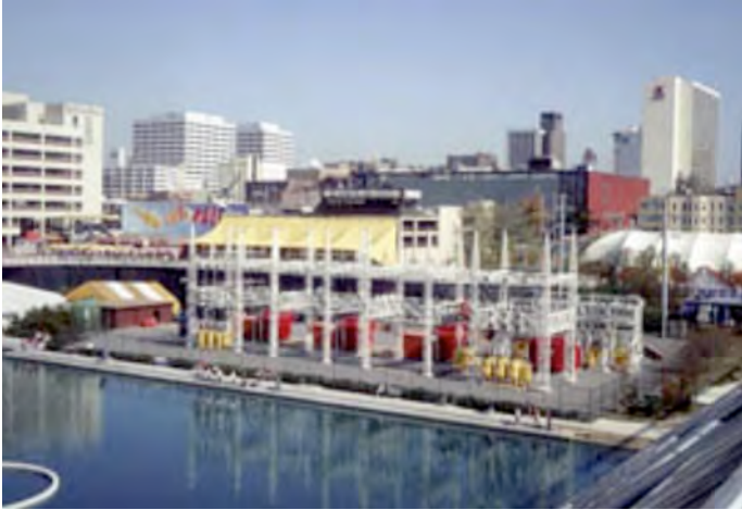
Substation decorated with paint
