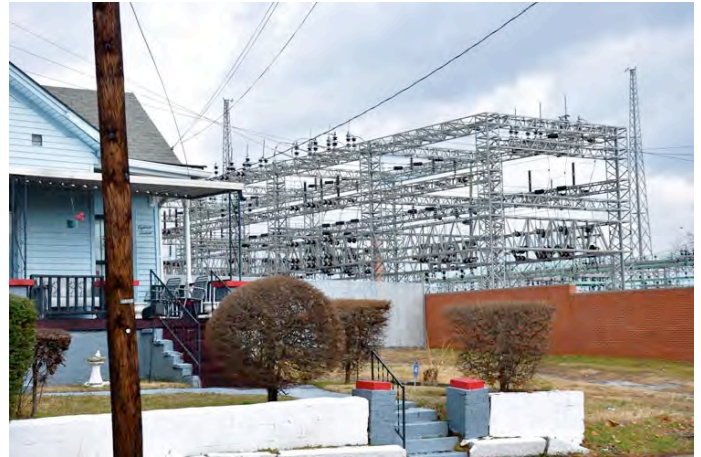
Substation located on Jo Johnston Avenue and Dr DB Todd Jr. Boulevard
