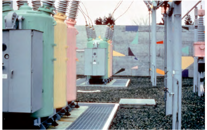
A background mural and painted components energize the substation
