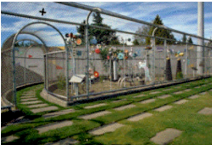
Protected walkway allows visitors to walk through the substation
