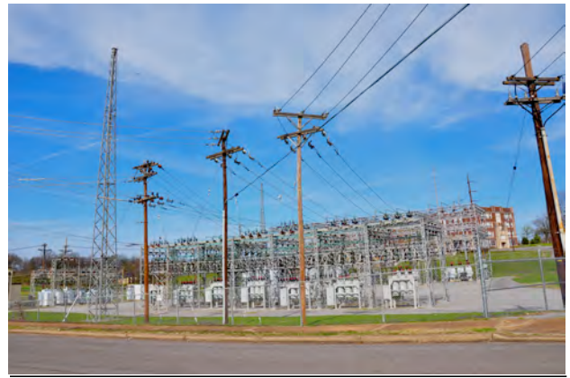
Substation located on Finn Street, behind East Nashville High School
