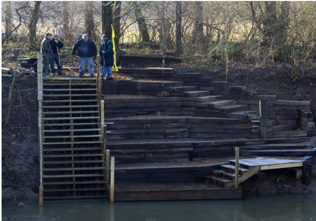
New structure for canoe access at the Rec Center just prior to final trim.
